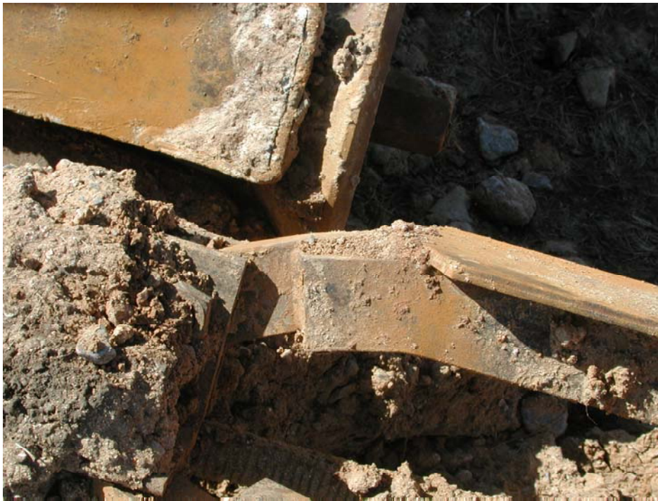
Figure 12: Picture of Slightly Bent Center Anchor after Removal
